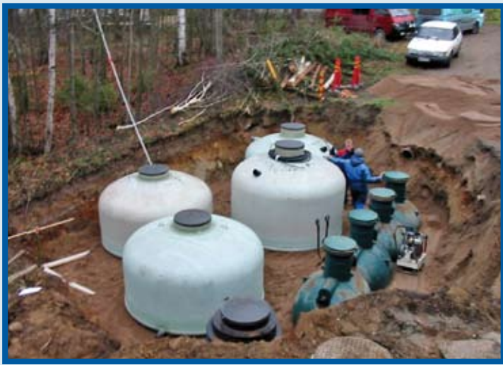
Photo 1 Showing the construction of a compact plant for two households in Kuusankoski, Finland. The picture shows the septic tank, two pre-filter tanks on the left and two tanks for phosphorus removal with Filtralite®P in the middle of the photo. The pre-filters are constructed with a recycling system.
